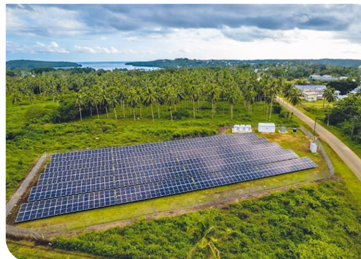
Solar array and battery energy system on Vava'u Island, Tonga.
