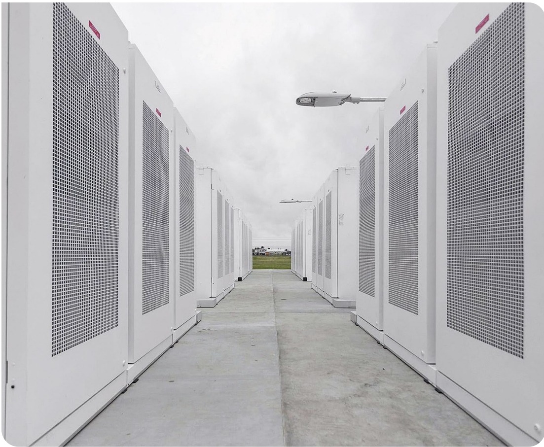
Cook Islands’ power utility company Te Aponga Uira’s Rarotonga BESS Project Airport South is a 2MW/8MWh Tesla Powerpack battery energy storage system.
